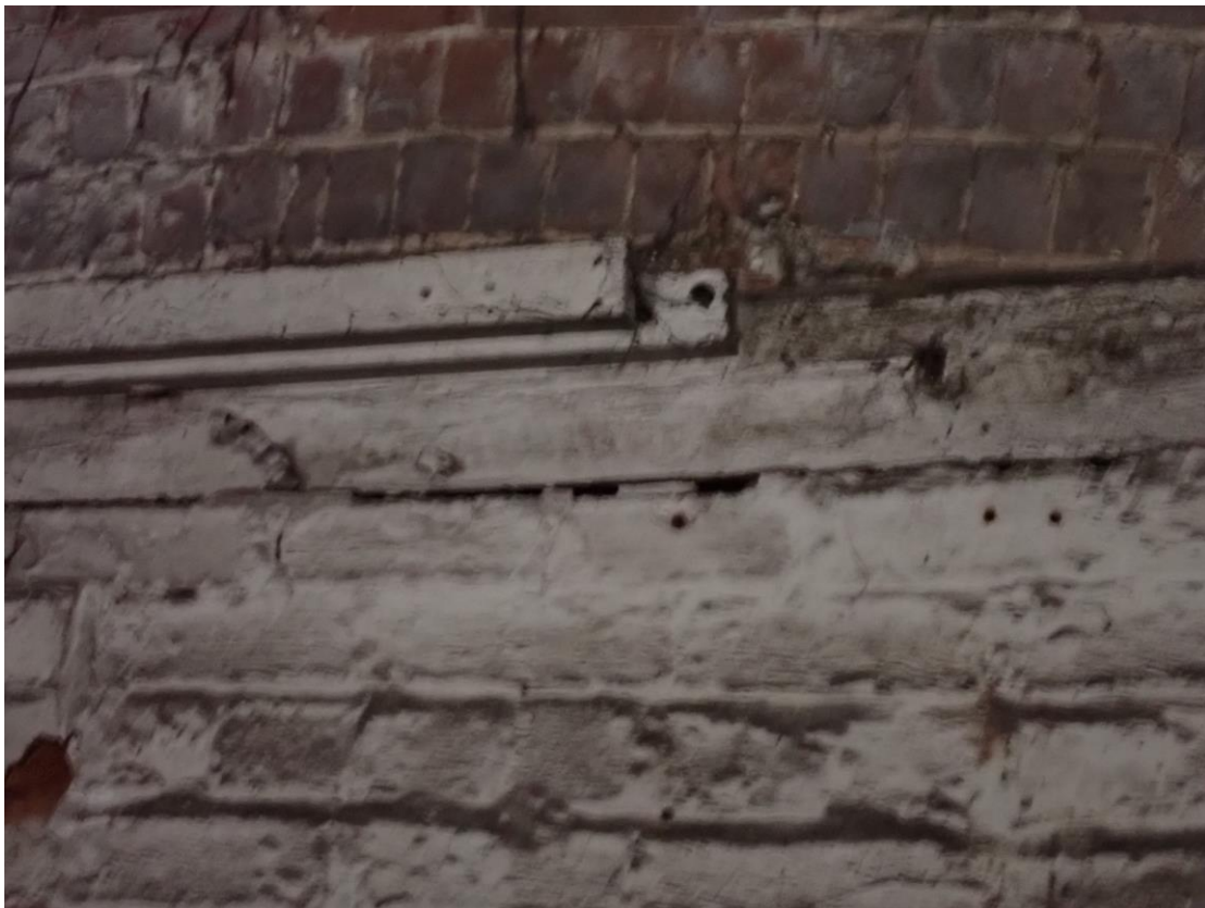
Photograph 16. Cavities between the timber and brickwork in Building 2.
