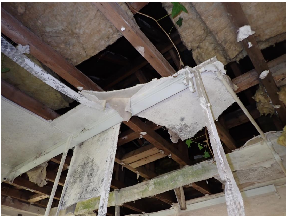
Photograph 20. Damage to the ceiling in the western extension of Building 3.
